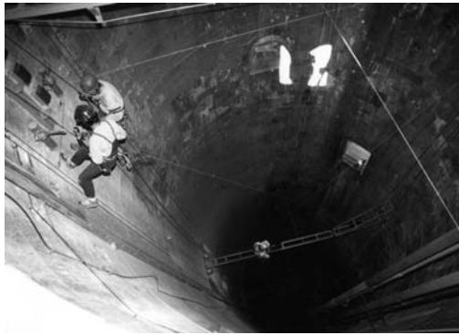
Fig. 3 – Measurements of relative displacement (automatic system). Long base extensometers with electrical transducers installed in the inner walls of the Leaning Tower of Pisa to measure the diametral and longitudinal deformations
